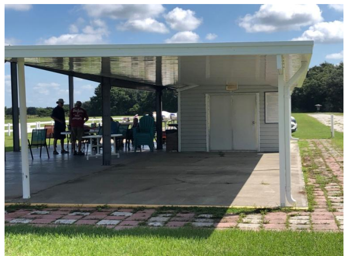
Thank you, Tim Dyal, for the new roof over our deck. Looks really good.
